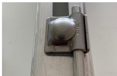
Anbindung Erdungsdraht an die C-Schiene Connection of grounding wire to the C-rail
