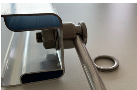
Anbindung Erdungsdraht an die C-Schiene Connection of grounding wire to the C-rail
